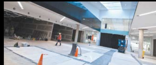
An impressive new light well has been installed in the main Myer entrance.
